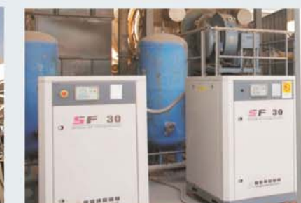
动力气源低噪声螺杆式空压机， 配置特制消噪室 Low-noise rotary screw air compressor with power source, equipped with a special noise cancellation room
