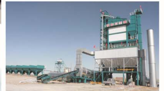
中铁十局4000型沥青混合料搅拌设备 4000 type asphalt mixing plant of China Railway No. 10 Engineering Group Co., Ltd.
