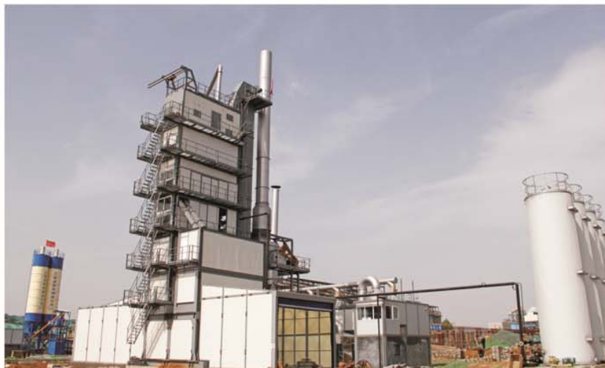
登封公路局4000H型沥青混合料搅拌设备 4000H type environmental asphalt mixing plant of highways agency, dengfeng
