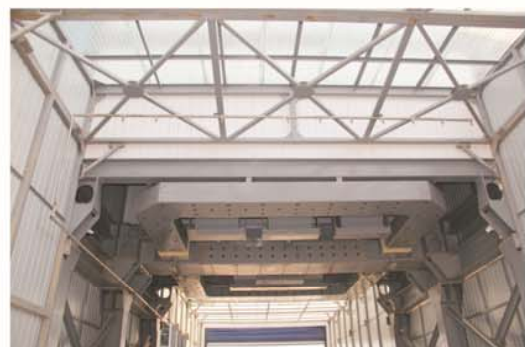
全封闭装车区 Full-closed loading area
