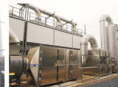
沥青烟处理系统 Asphalt fume treatment system
