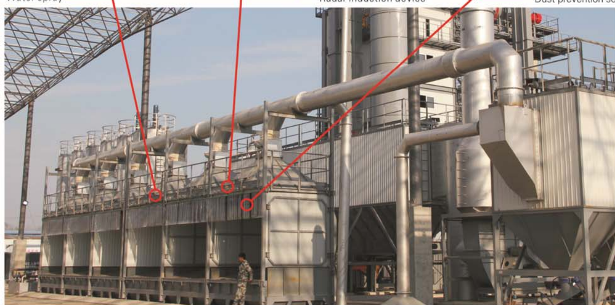
雷达自动感应抽风系统、半下沉或地垄式结构 Radar automatic-induction exhausting system and half sinking or ridge type structure
